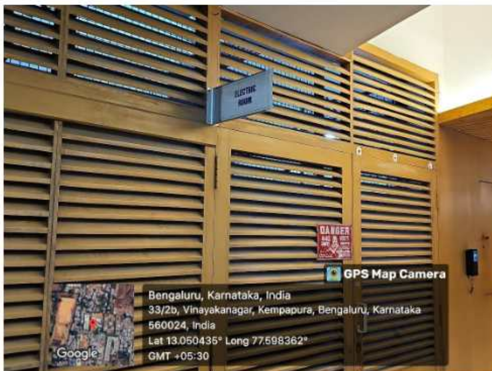
Dedicated Electric room
